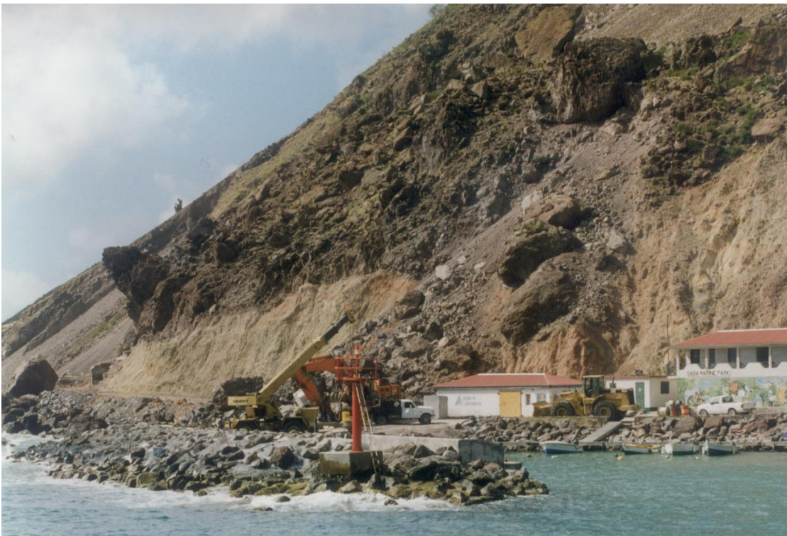
Figure 1 : Landslide in the harbour of Fort Bay of February 1997.
